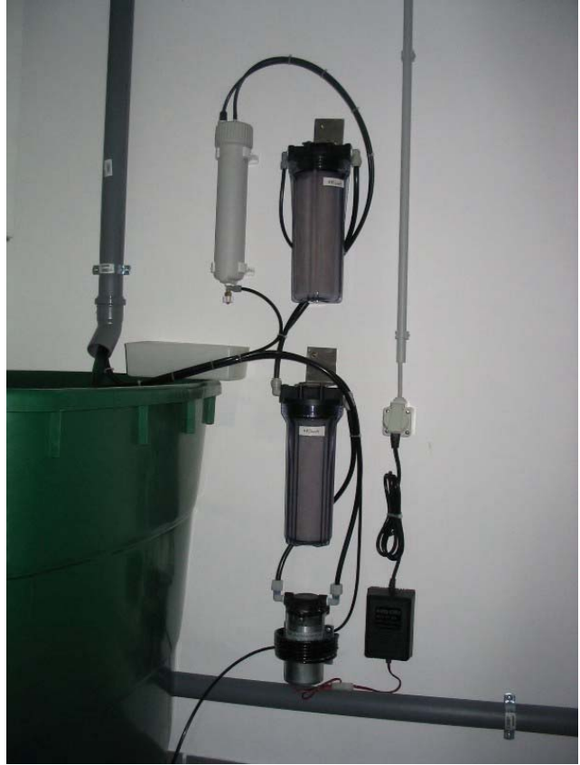
Pumpe, Filter, Membrane
