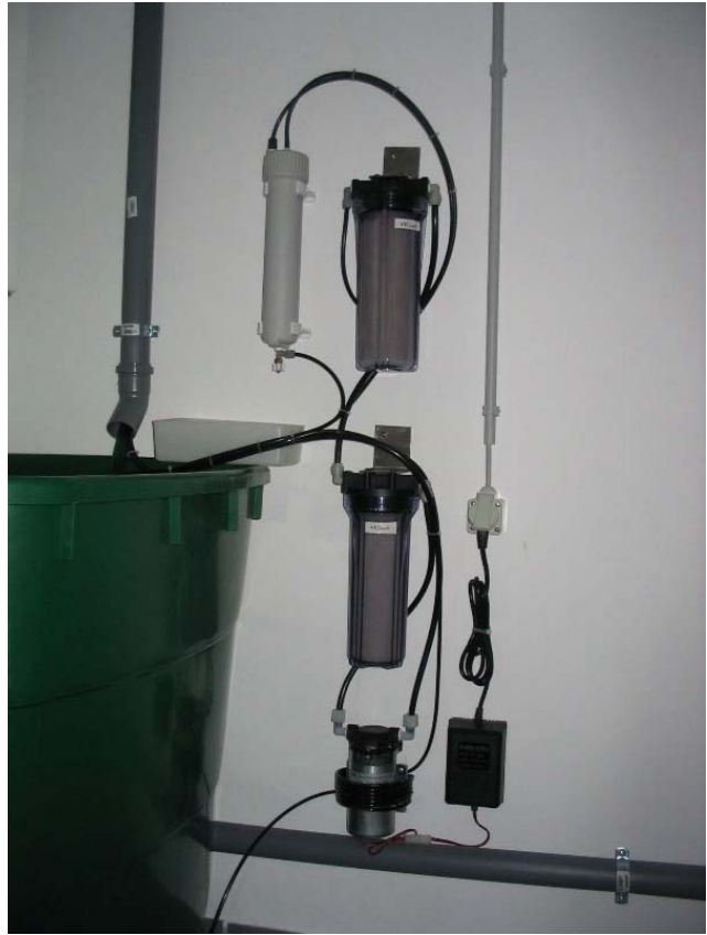
Pumpe, Filter, Membrane
